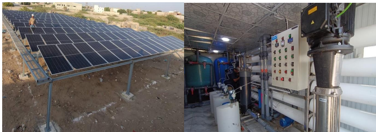
The installed water desalination in Al-Hoedeutah governorate.
