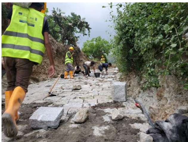
A road being rehabilitated through short-term employment opportunity in Najrah district, Hajjah.
