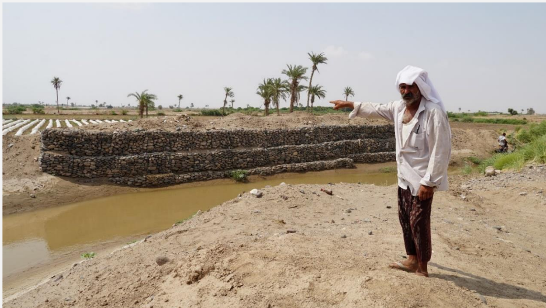
Mohammed Ali, a farmer from Lahj Governorate, points to the newly constructed gabion.
