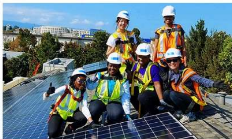
Installation of roof top solar PV panels in Palo Alto as part of the Techwomen Professional Exchange Program, San Francisco (CA, USA), October 2018.
