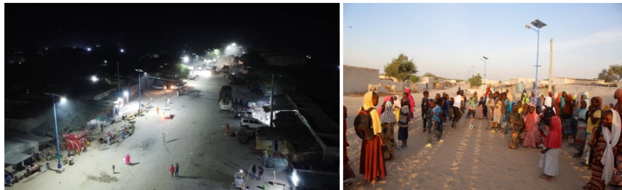
Solar-powered streetlights (Left: Far North, Cameroon | Right: Tam, Niger) © UNDP Cameroon | © UNDP Niger
