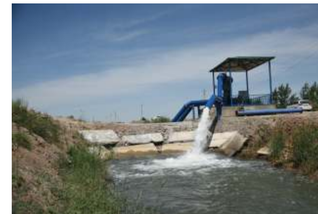
The water is delivered into local irrigation canal from newly built by the UNDP/GEF project energy-efficient pumping station. Photo: UNDP
