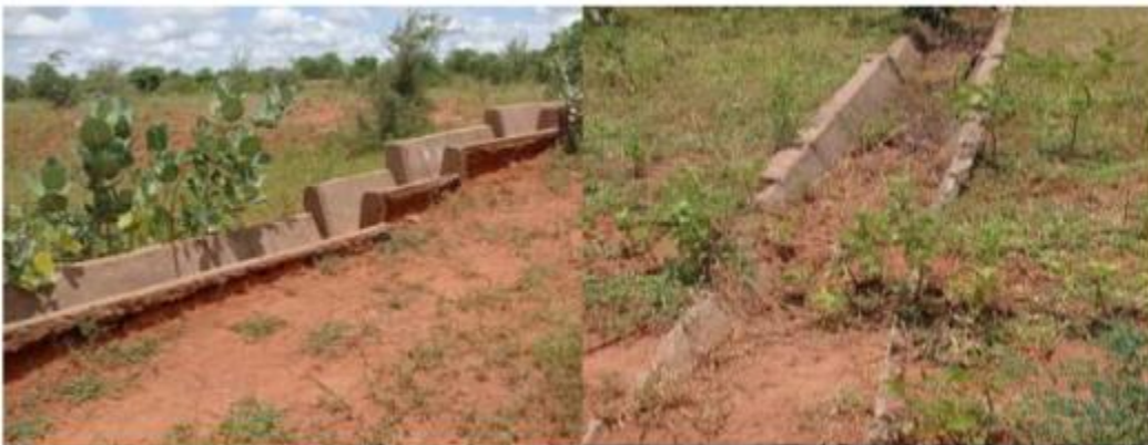
Plate 7 Damaged infield canals
