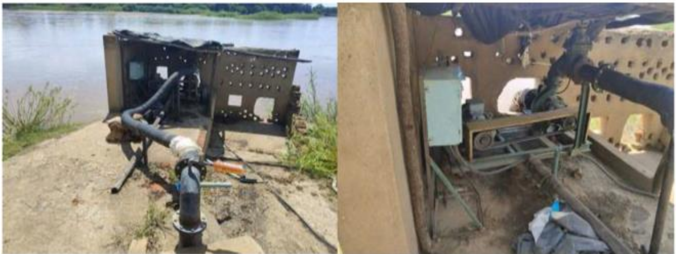
Plate 12: Centrifugal pump on the banks of Save River
