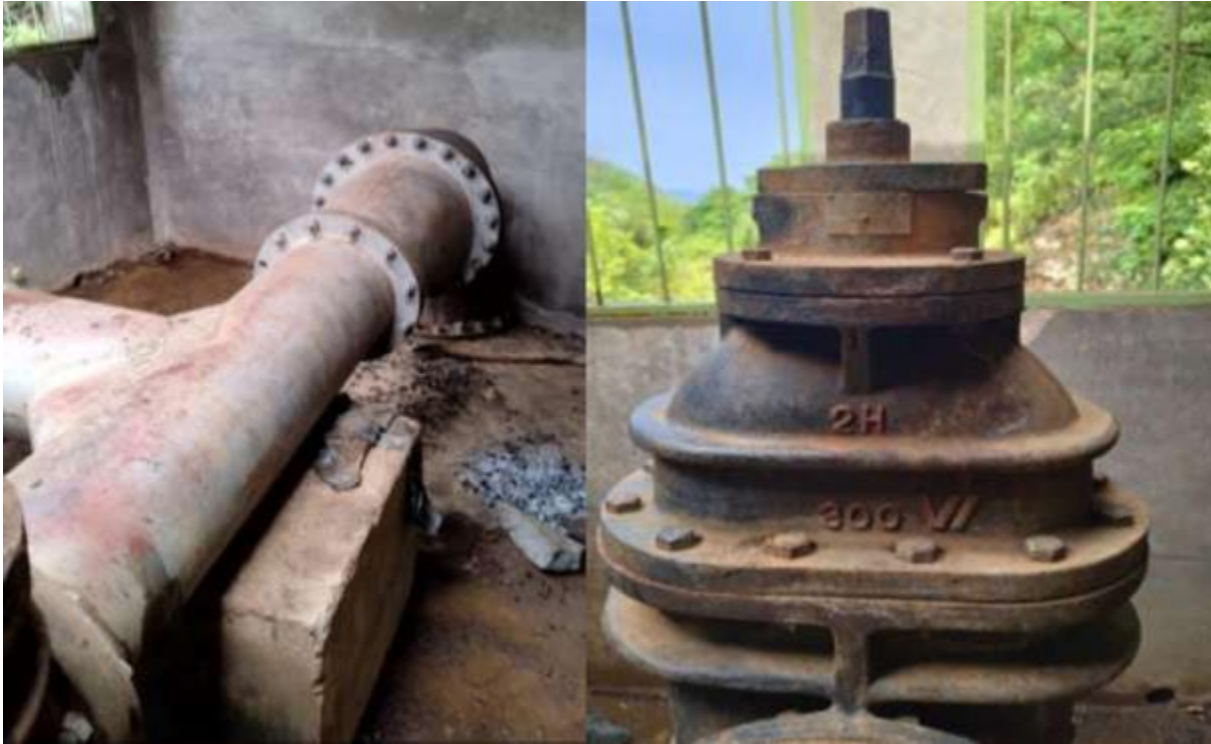
Plate 2: Outlet pipe and control valve
