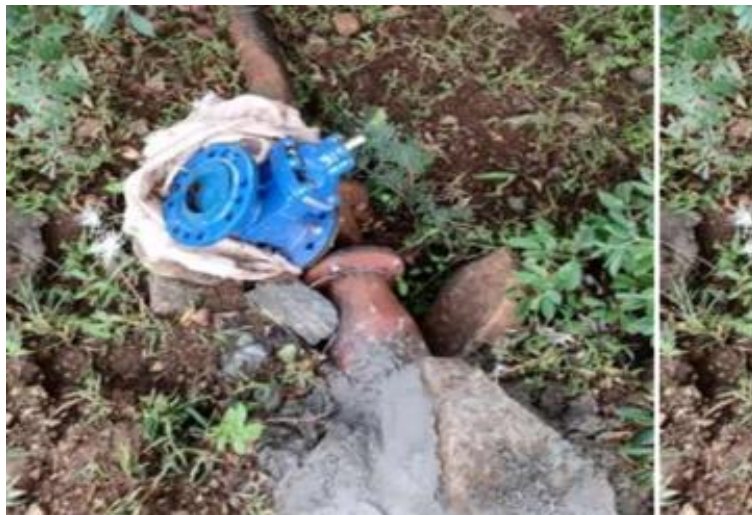
Plate 5: Scour Valve on 100mm Dia Steel Section
