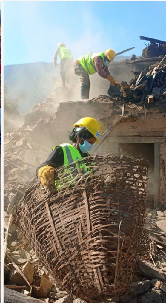
A female community member engaged in debris removal using cash for work at Aathbiskot Municipality, December 2023. © Ganesh Bishwokarma/UNDP Nepal
