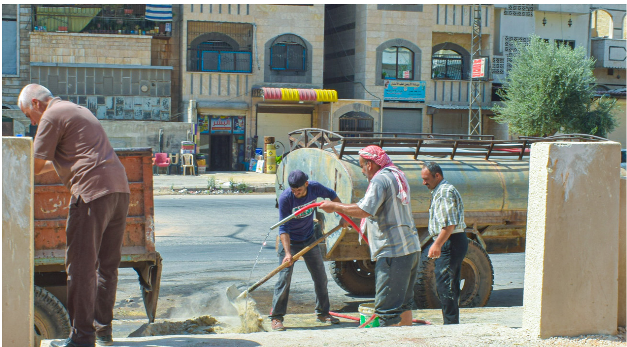
Image depicting the community's participation in the completion of the rehabilitation works of Al-arbeen Public Park
