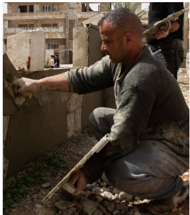
Field visit to supervise the implementation of the construction work of the garden fence by the local community and the volunteer committee in Al-Fayhaa neighborhood
