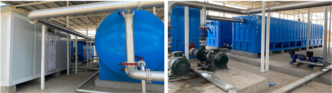
Rehabilitation of Al-Bo Faiadh Water Treatment Plant (WTP) in Yathrib, Salahaldin governorate
