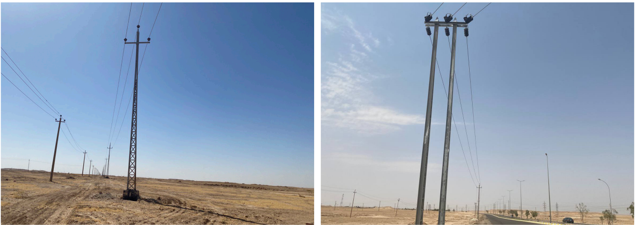
Rehabilitation of the Main Electrical Feeder from Anah Electrical Substation to Al-Sakrah District in Anbar
