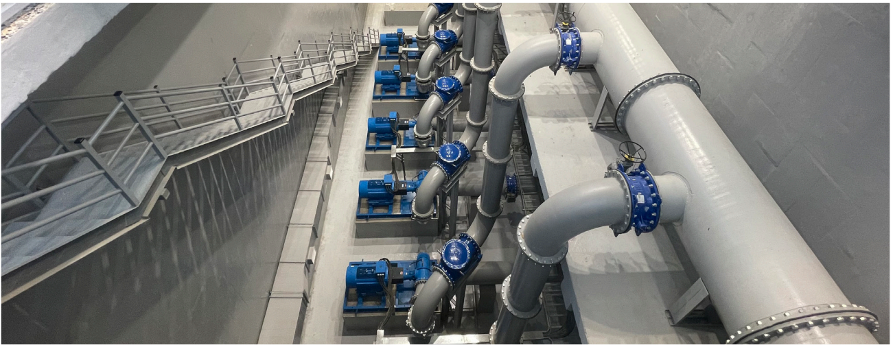
Fallujah Stormwater Lift Station - Installed pumps and mechanical fittings
