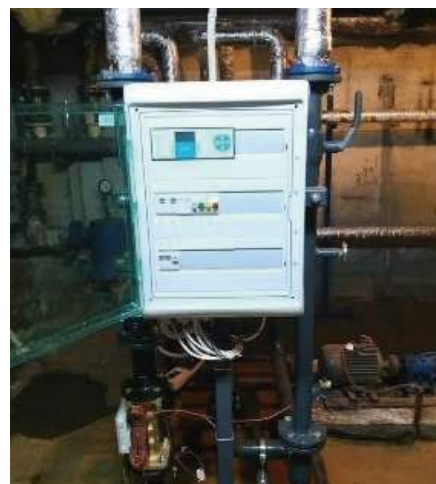
Picture 29. Control cabinet for IHS SynergyData
