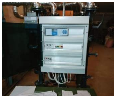
Picture 21. Control cabinet for IHS SynergyData
