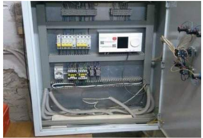
Picture 3. Control cabinet Danfoss
