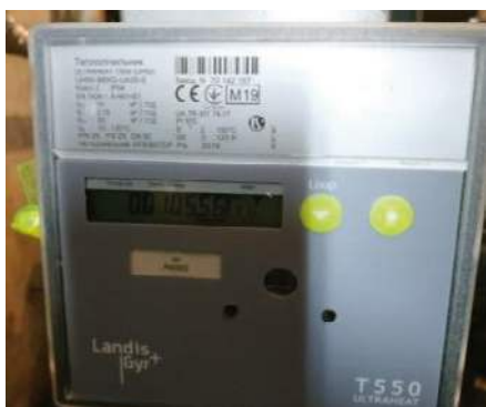
Picture 19. Heat meter Ultraheat
