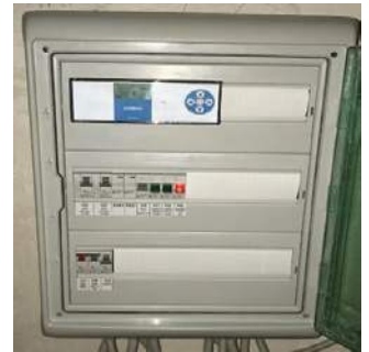
Picture 12. Control cabinet for IHS SynergyData
