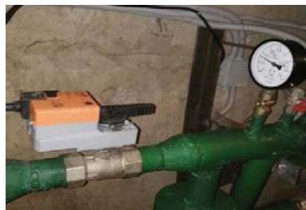
Picture 38. Temperature controller Belimo
