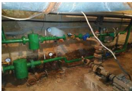
Picture 36. Heat carrier regulation system and heat meter
