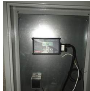
Picture 11. Heat meter Sempal
