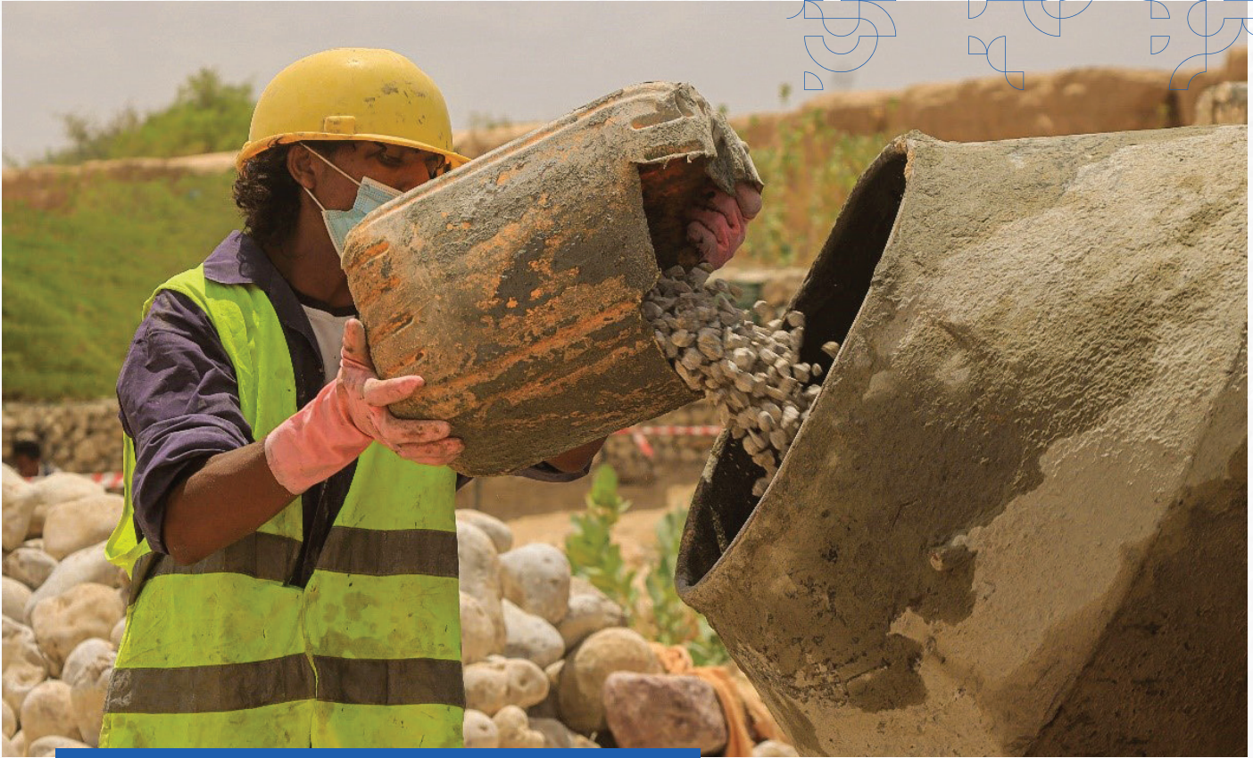
Muhammad Saleh, 22, works on the construction of irrigation channels and water barriers through a wage employment scheme. Photo Credit: UNDP Yemen / 2022
