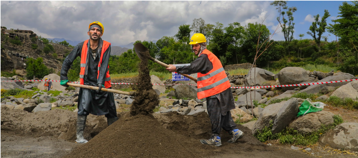
These laborers are working on a flood wall in Dara-i-Noor, Nangarhar province. This protects the community from the impacts of climate change and provides valuable cash-for-work opportunities.
