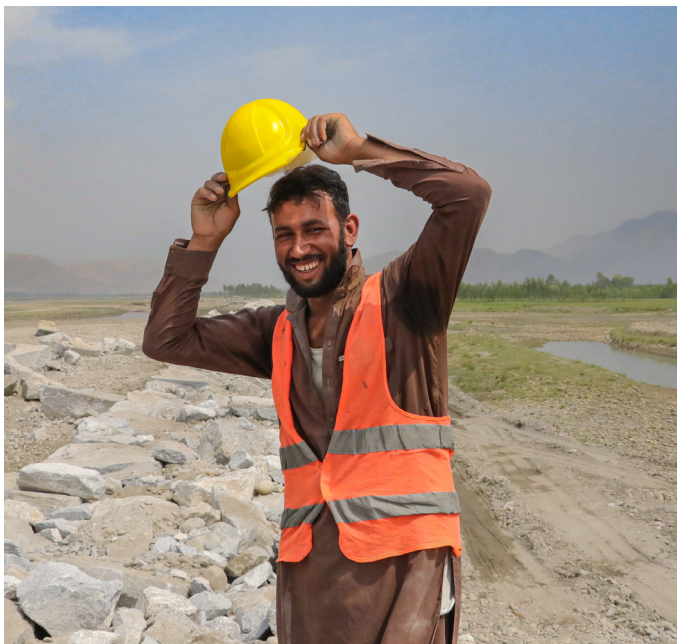
A big smile from Ahmadullah as he works on a protection wall in Nangarhar province. This crucial infrastructure project aims to safeguard communities, homes, and farmlands from the destructive impact of seasonal flash floods and rising river waters. Ahmadullah's efforts symbolise the resilience of local residents and their determination to protect their livelihoods and create a safer environment for future generations.
