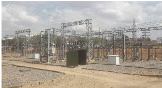
Photo 8: TANESCO Power Station in Tabora
