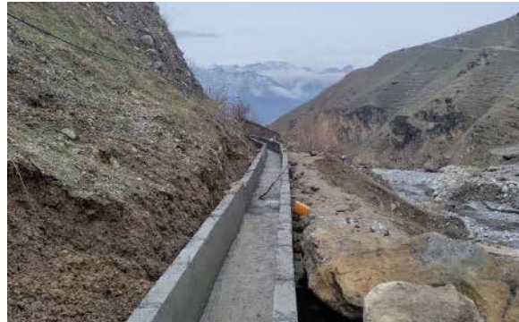
Irrigation canal construction in Badakshan province, North-eastern region. Livelihood Promotion in Tajik Afghan Cross - Border Areas (LITACA-III)
