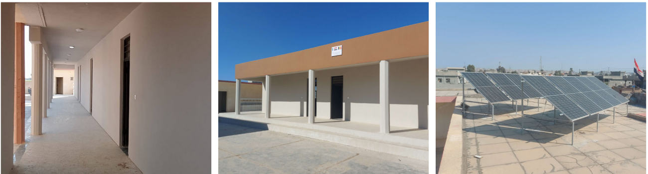
Construction of classrooms for Al Adnania Secondary School in Suleiman Bek, Salahuddin Governorate
