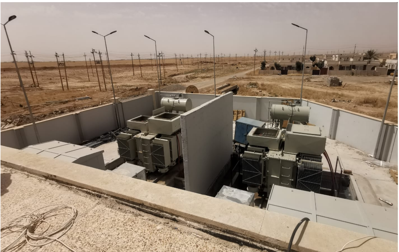
33/11.5 kV 10MVA Substation in Sinjar-Domez
