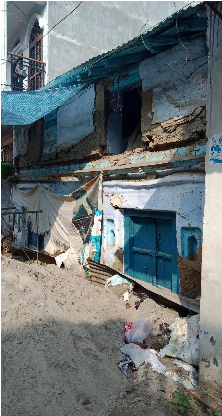
Figure 18 Narrow and unmanaged road with risky houses, Eklaini Bazar, Nepalgunj
