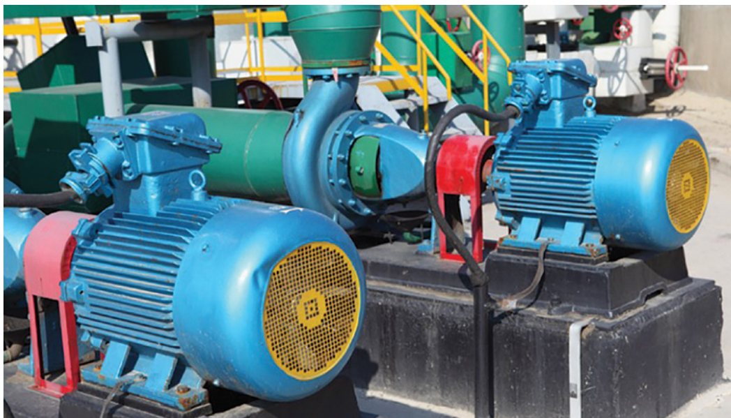
Energy efficient pumps
