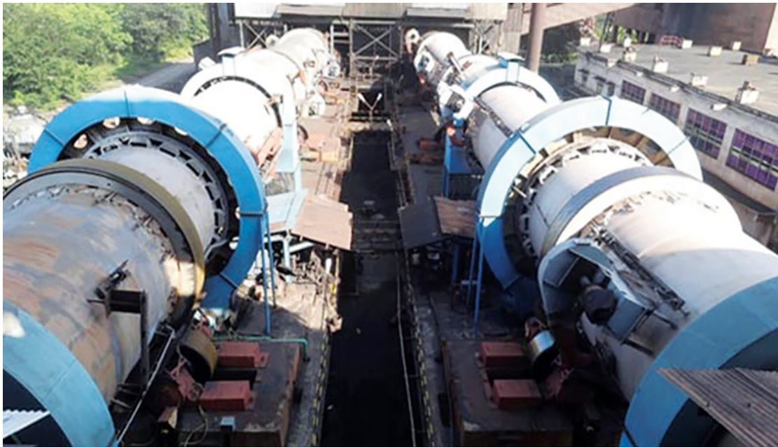
A two-kiln DRI plant
