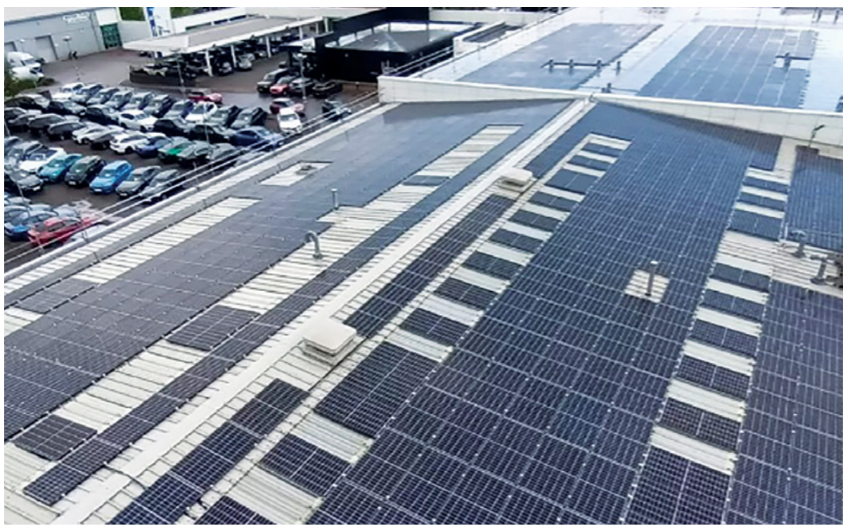
Rooftop solar PV system
