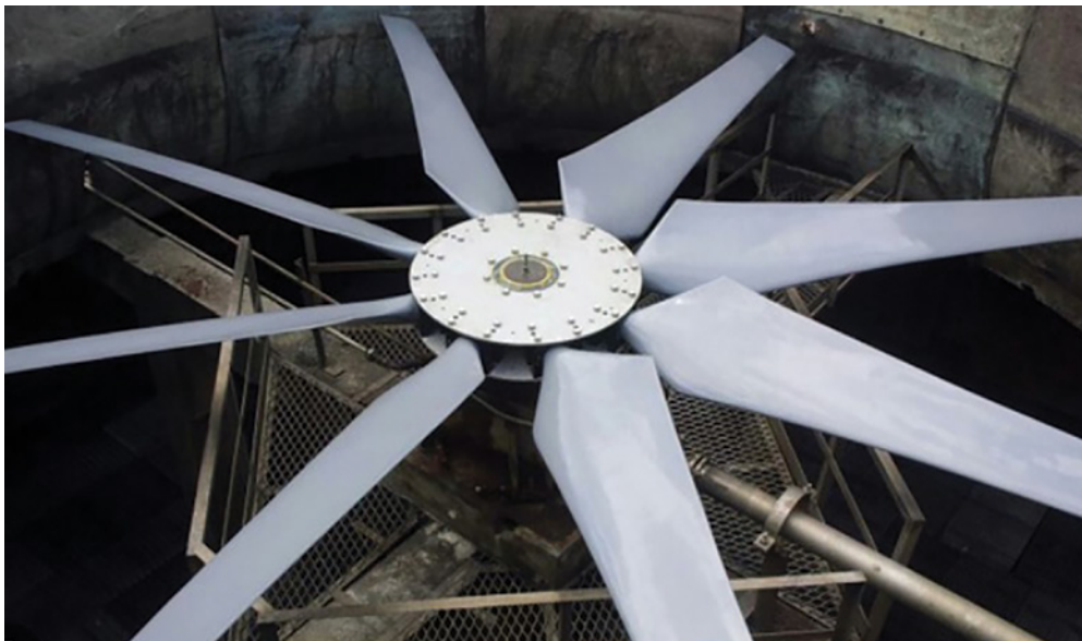
FRP blade in cooling tower
