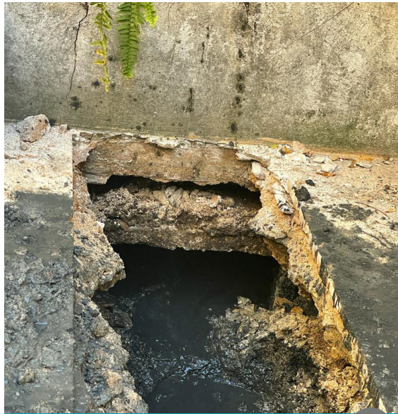
Blocked open sewer manhole
