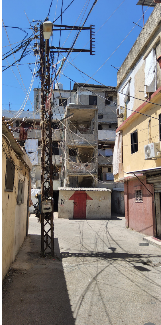
Ad-hoc electricity connections
