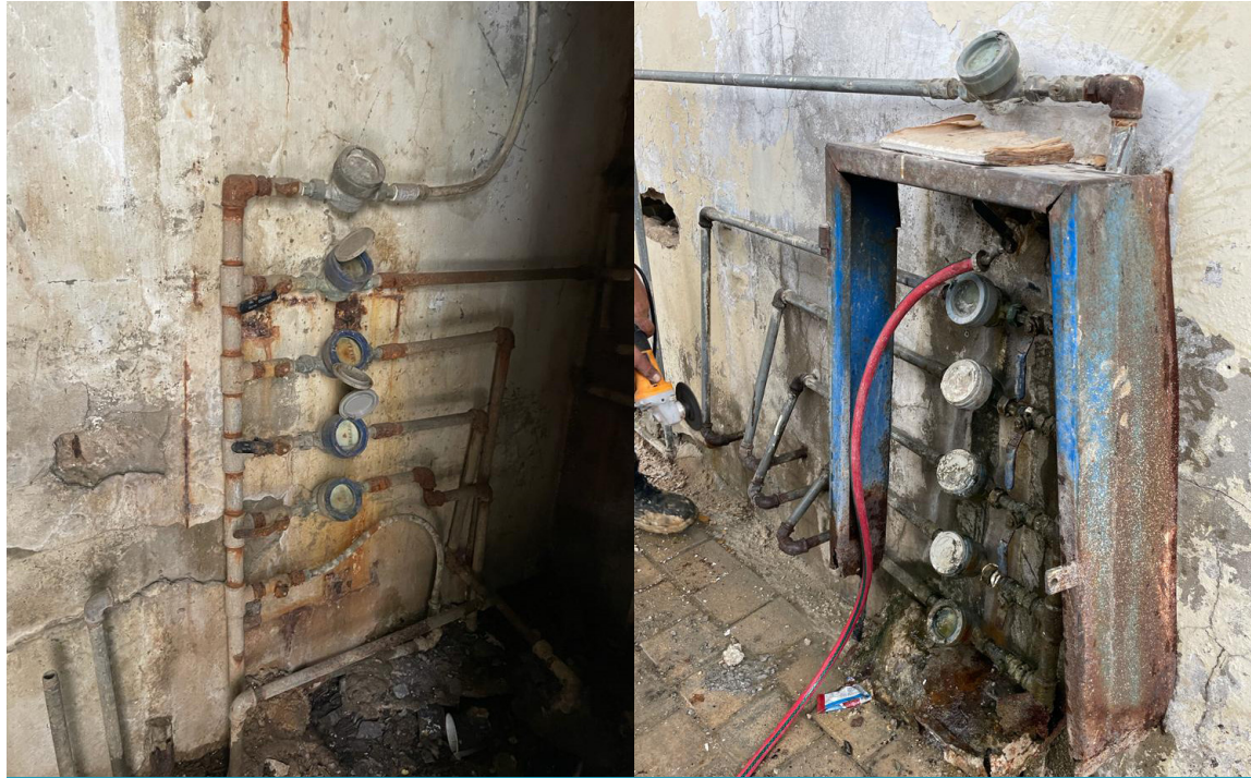
Corroded manifolds with non-functional meters
