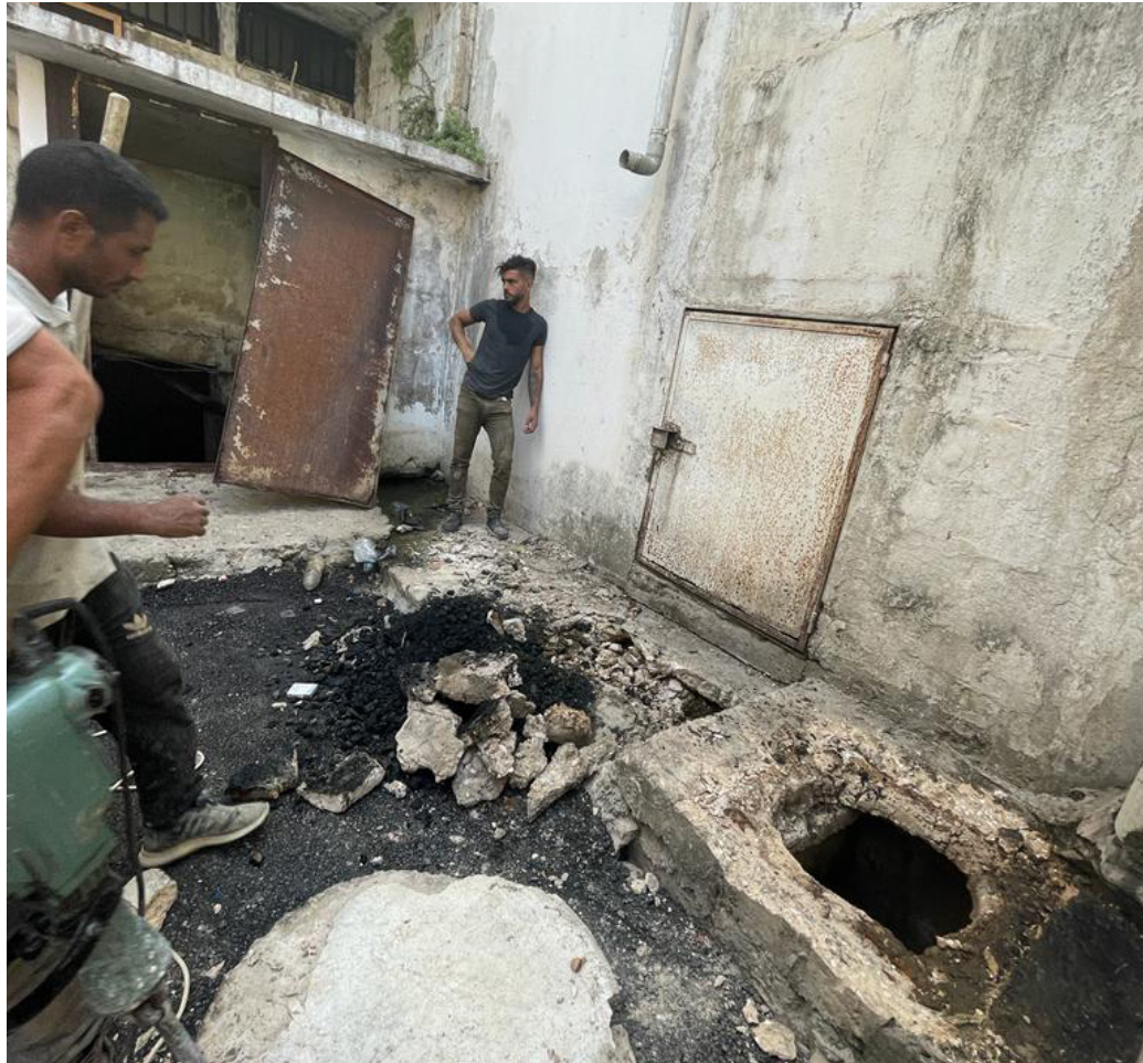
Broken blocked manhole
