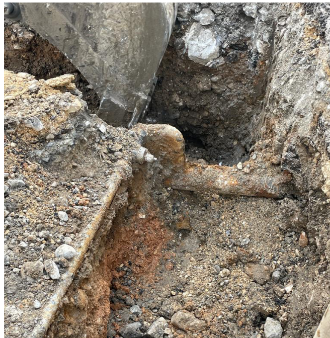
Corroded water pipe
