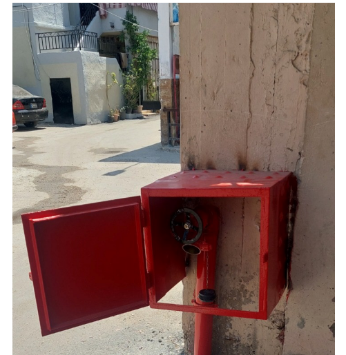
Installed street fire hydrants
