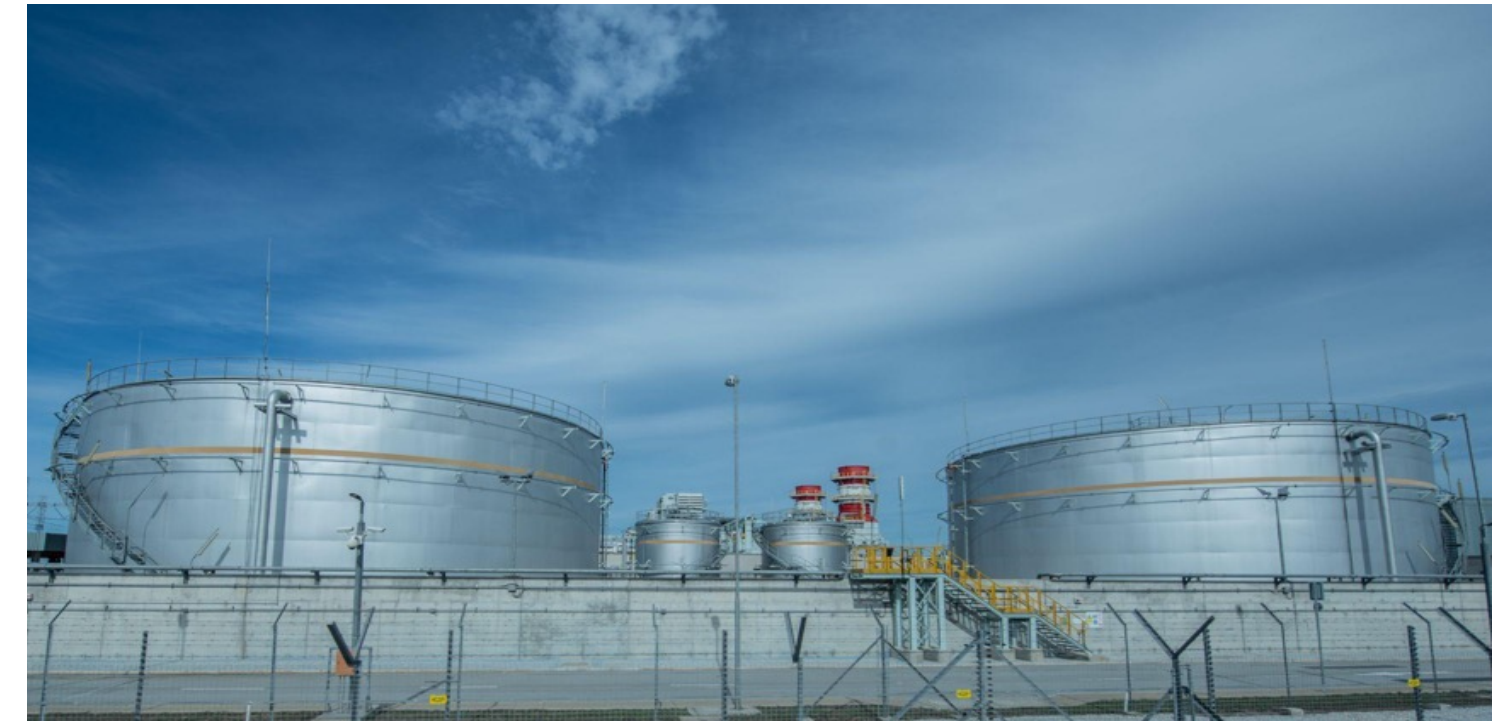
Image 6. The Dedisa Peaking Power Station in Ngqura, a 335MW open cycle gas turbine (OCGT) peaking plant.
