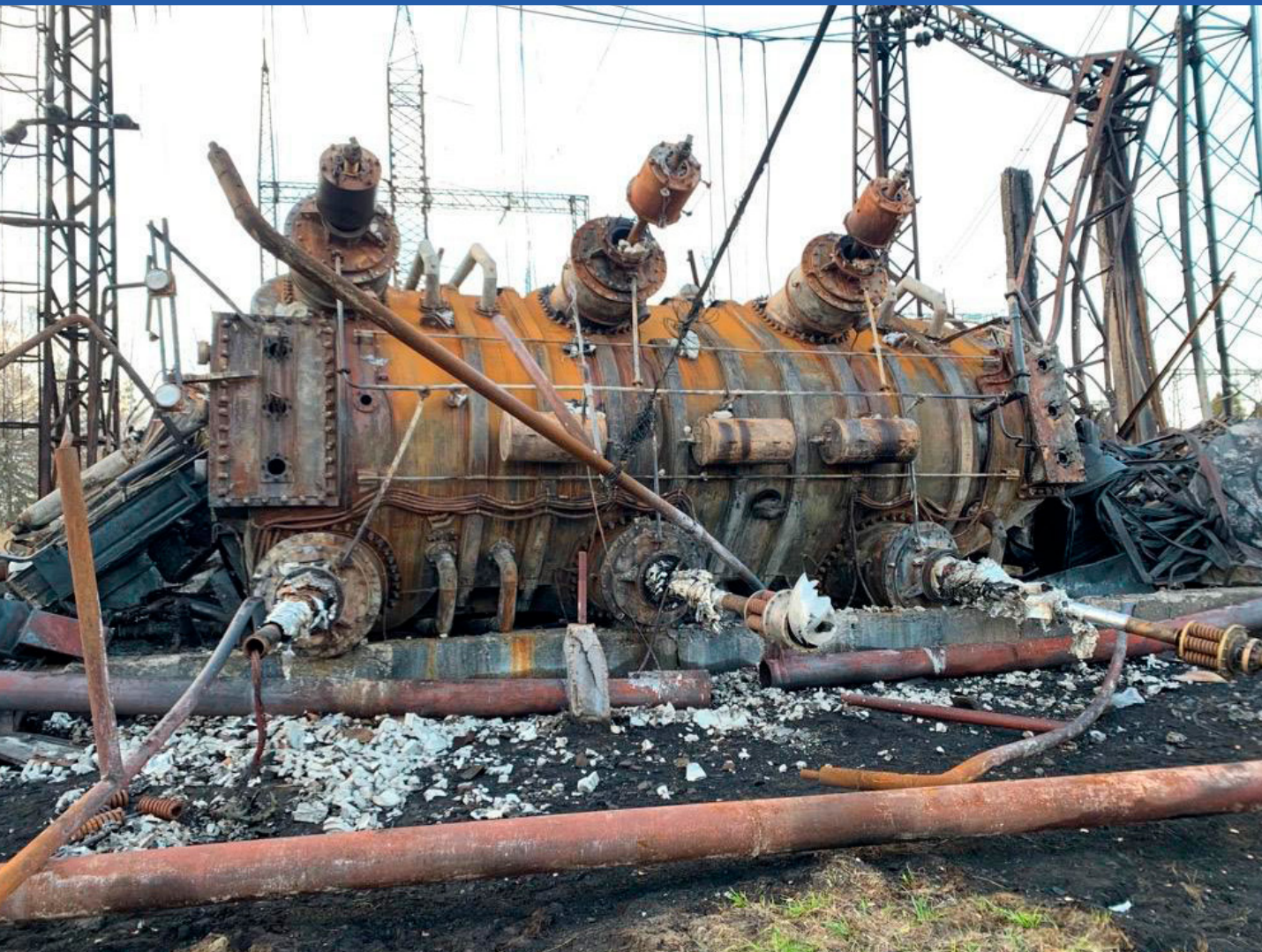
Completely destroyed 330kV 200M VA auto-transformer
