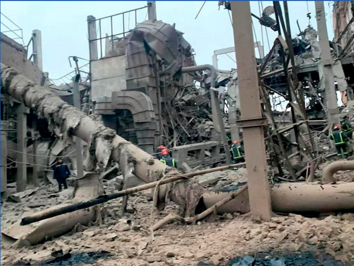
Completely destroyed combined heat and power plant
