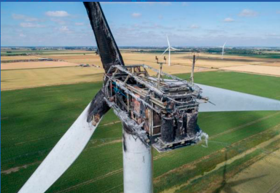
Damaged wind power plant
