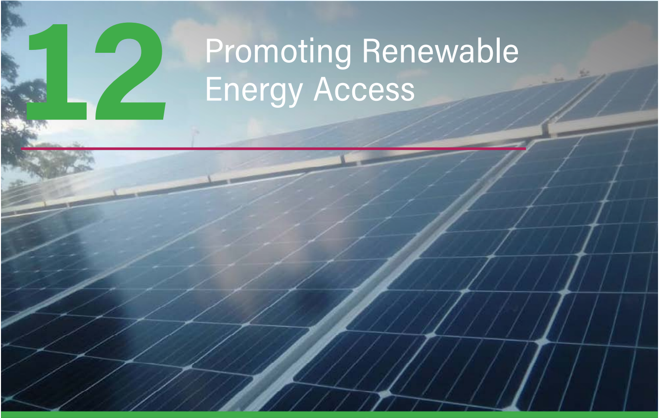
PHOTO: Solar PV installation at Rukunyu Health Centre IV in Kamwenge district. ©UNDP Uganda
