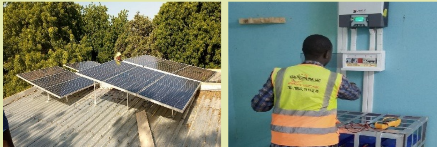
Installation of solar kits at the maternity hospital of Seytenga and Falagountou, Commune of Seytenga, October 2022
