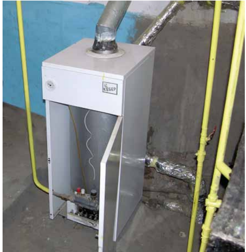
Photo 7. An energy efficient water heating gas boiler with automatic regulation of gas supply, installed at the "Baymukhamedov" rural health clinic.
