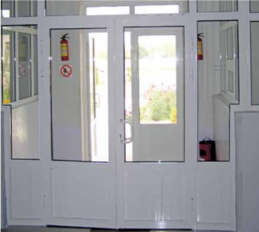
Photo 10. Arrangement of a tambour (lobby), installed to reduce heat loss in the “Baymukhamedov” rural health clinic, Tashkent region.
