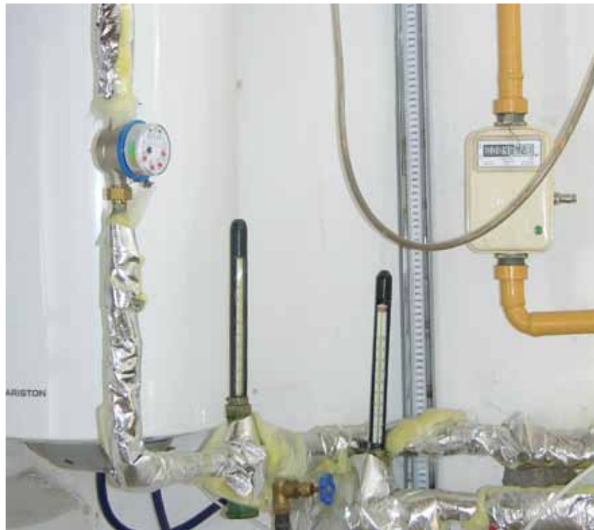
Photo 11. Some of the meters installed at the “A. Umarov” rural health clinic, Tashkent region.
