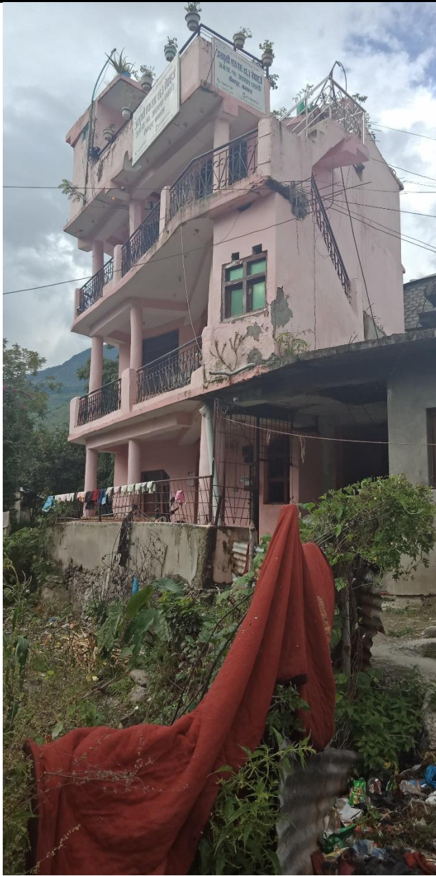
Figure 14 Safety Walk - Building seems risk in earthquake, Jayaprithvi
