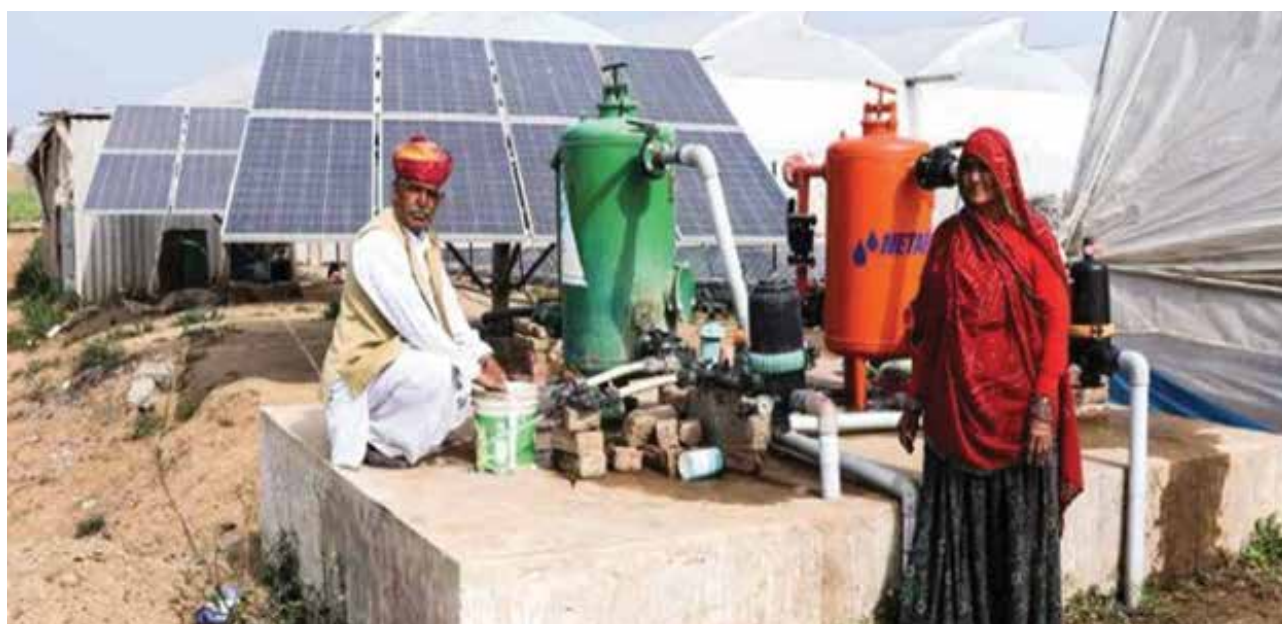
A 5 horsepower solar pump installed in Sambhar, Jaipur district, Rajasthan. Source: MNRE Annual Report.
