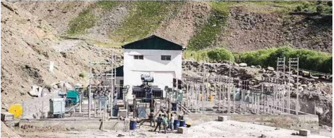
1.5 MW Sangrah SHP in Kargil District under Ladakh Renewable Energy Initiative, MNRE Annual Report
