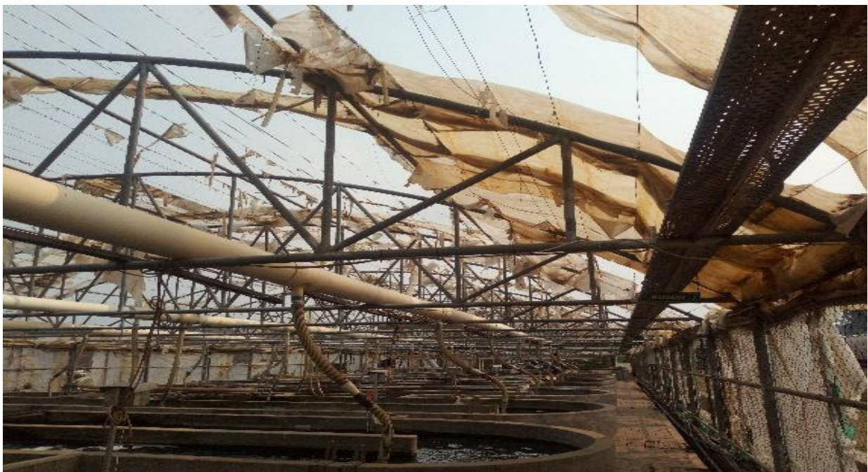
PLATE 1: Greenhouses are used to adapt to extreme low temperatures which affect fish growth. Heavy winds have destroyed the structure.
