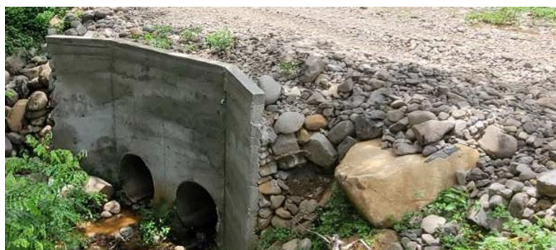
Culvert and Headwall put in place as risk measures, Ba, Fiji (photo by MRMDDM)
