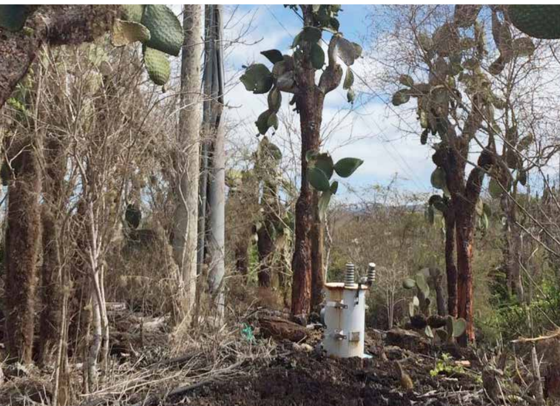
REPLACEMENT OF PCB CONTAMINATED TRANSFORMER (ISABELA, GALAPAGOS). PHOTO BY ECUADOR PCB PROJECT
