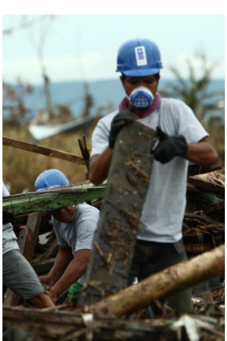
Workers supported by a UNDP Cash-for-Work programme clear rubble from different sites affected by Typhoon Haiyan. Photo: UNDP Philippines
