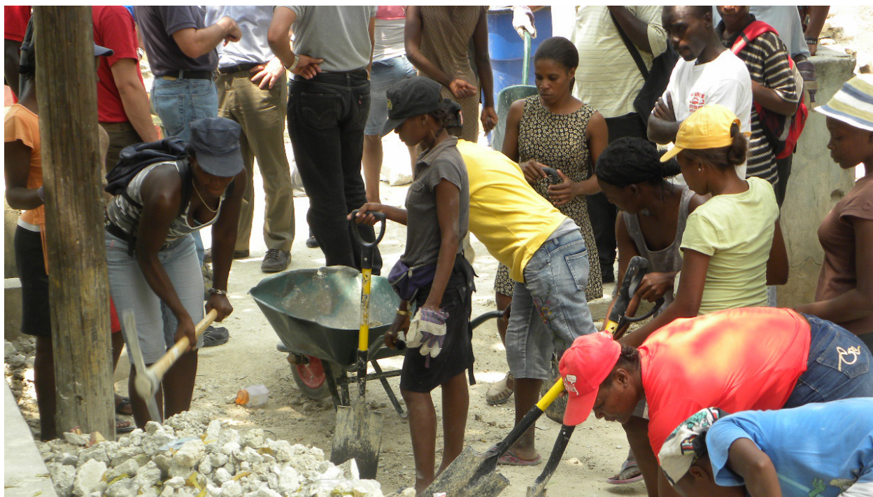
Haitian men and women work in tandem in Fort National, Port-au-Prince, in order to complete the arduous task of shifting debris generated by the 2010 earthquake, sometimes one piece at a time, to a temporary collection site, before the debris is transported to recycling or dumping sites. Photo credit: UNDP Haiti.
