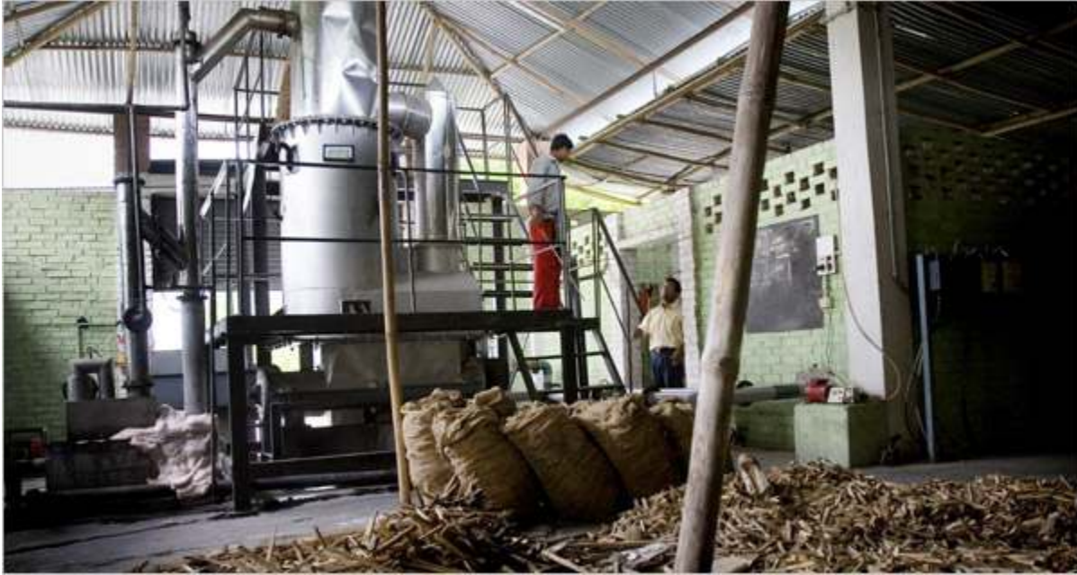
A generator fueled in part by biomass in Baharbari, India.
