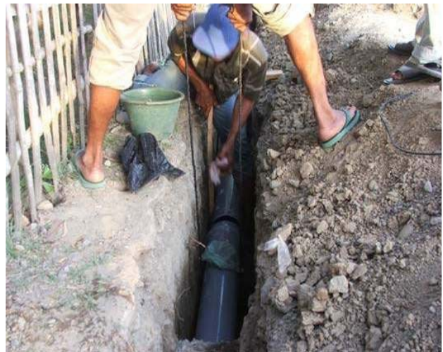
The laying of water transmission pipes in Rawa Gampong, Pidie District, Aceh, Indonesia. Work is underway to connect this remote tsunami-hit area to a sustainable supply of clean water.
